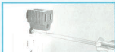
Use one of the wall receptacle screws to ground an adapter to the outlet metal box.
